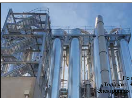
Multiple effect evaporation plant
